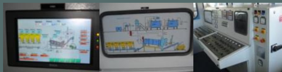
*** PLC TOUCH SCREEN TYPE PANEL
